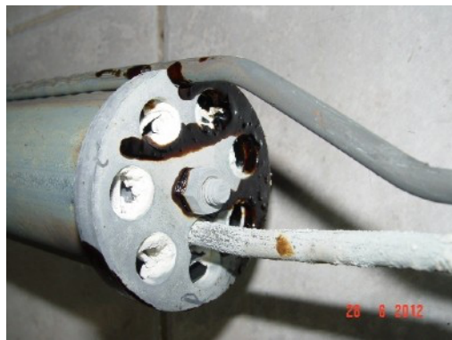
Mineral deposits on an electrode permanently damaged by lack of acid cleaning
